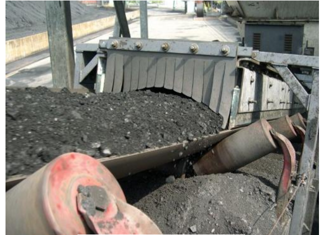
Figure 2: Coal Spillage from Conveyor
